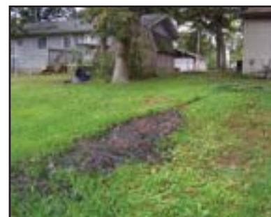
Failing Septic Systems in LaPorte County
